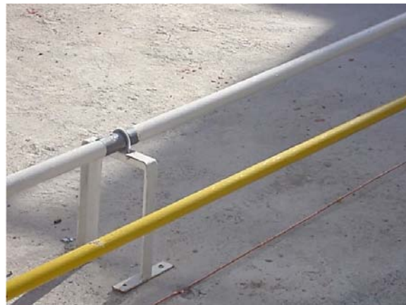
Figure 5. Signaling of LPG pipes (yellow LPG vapor, white LPG liquid).
