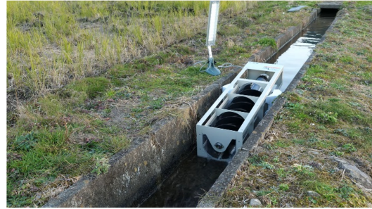
Figure 11. Microhydraulic generation system installed in a stream
